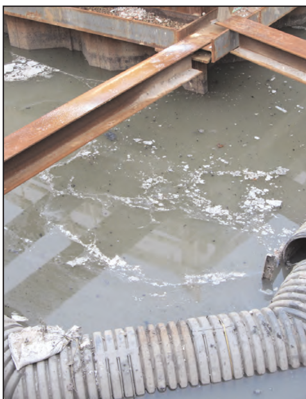
Fetid water was left untended for over a month as the city stopped paying the contractor (photo by Fiala).
